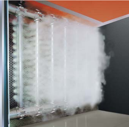
In-duct steam humidification
