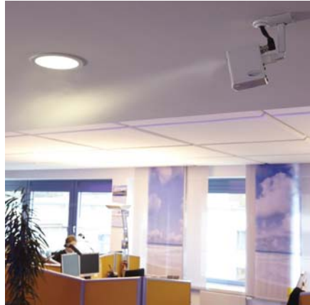
In-room spray humidification
